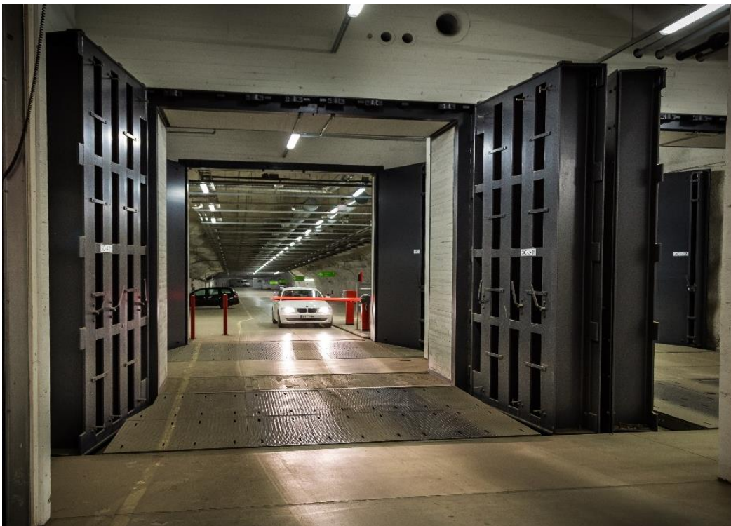
Heavy 4,4m x 4,5m Double Leaf Doors installed at the entrance of an underground car park.
